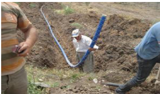
Work in progress to provide clean potable water in Dahuk through an ERF-funded project targeting 320 beneficiaries.
