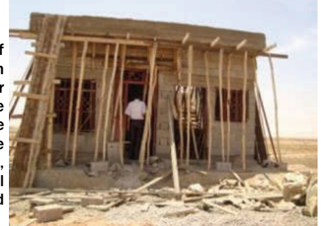
CHF constructs a small house for a civilian victim of conflict as part of USAID CAP III's Marla Ruzicka Iraqi Victims of War Fund
