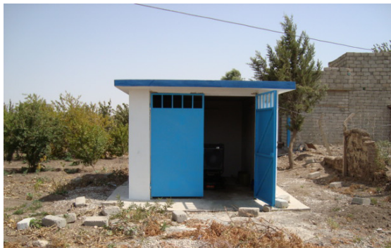
Generator Room / Zavi Rash Village / KURDS
