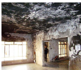
Falluja Shelter Damages April 2009
